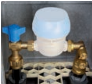
43 Z Before water meter valve lockable + check valve (elbow)
