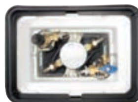
F45 K before water meter valve tamper-proof K + valve- check valve 518C (elbow)
