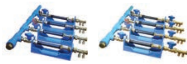
Fitted rails mounted on manifolds for multiple metering equipment
